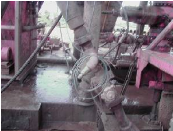
Picture.1 Pressure sensor installed on the choke manifold to receive pulses containing data sent from downhole
