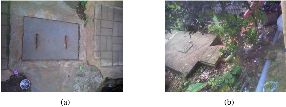
Figure 3. The condition of: (a) Inspection chamber no.2; (b) inlet of the septic tank
