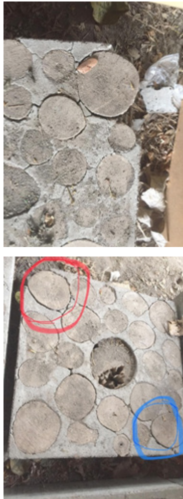
Figure 5. Condition of the top side of the floor block after 5 months
