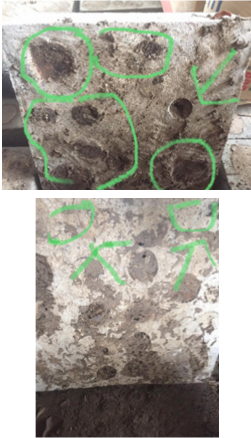
Figure 3. Condition of the bottom side of the floor block after 5 months
