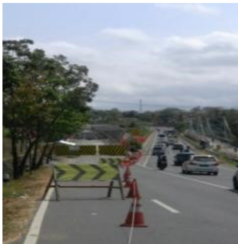
Figure 16. Construction of Progo Bridge in Sentolo Subdistrict that connects between Bantul, Sleman and Kulonprogo districts
